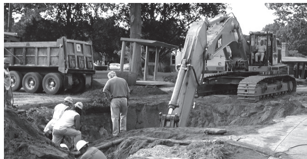
Starting next month, digging begins on the first of 110 miles of sewer pipe trenches for Chatham's Big Dig.
